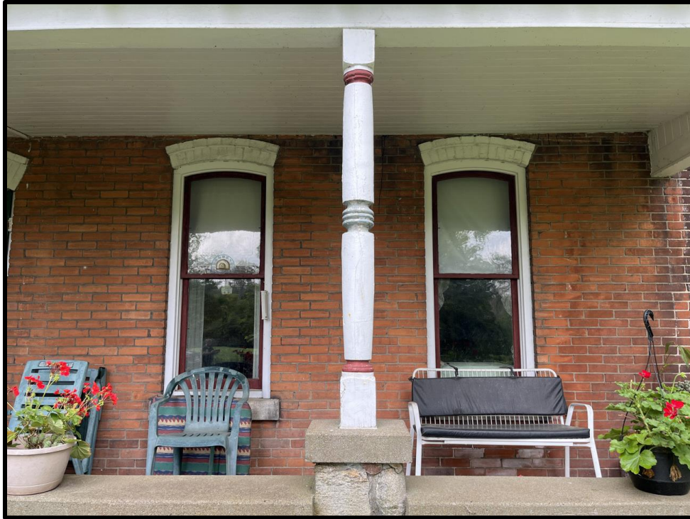
Image 3: Detail of Window Openings on Façade of 5187 Sherkston Road (Photo taken on July 21, 2023; Facing Southwest)
