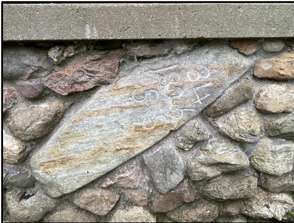
Image 2: Detail Ordnance Stone in Front Porch Wall (Photo taken July 21, 2023; Facing Southwest)
