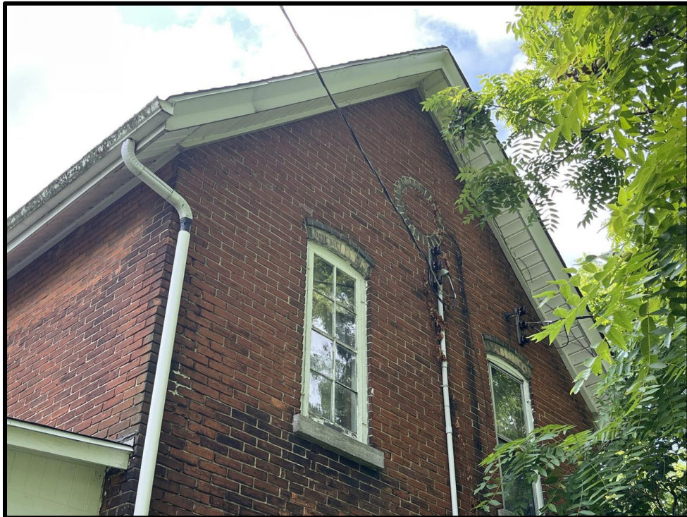
Image 20: Detail of Buff Brick Round Feature in Northwest Elevation Gable End of 5187 Sherston Road (Photo taken on July 21, 2023; Facing Southeast)
