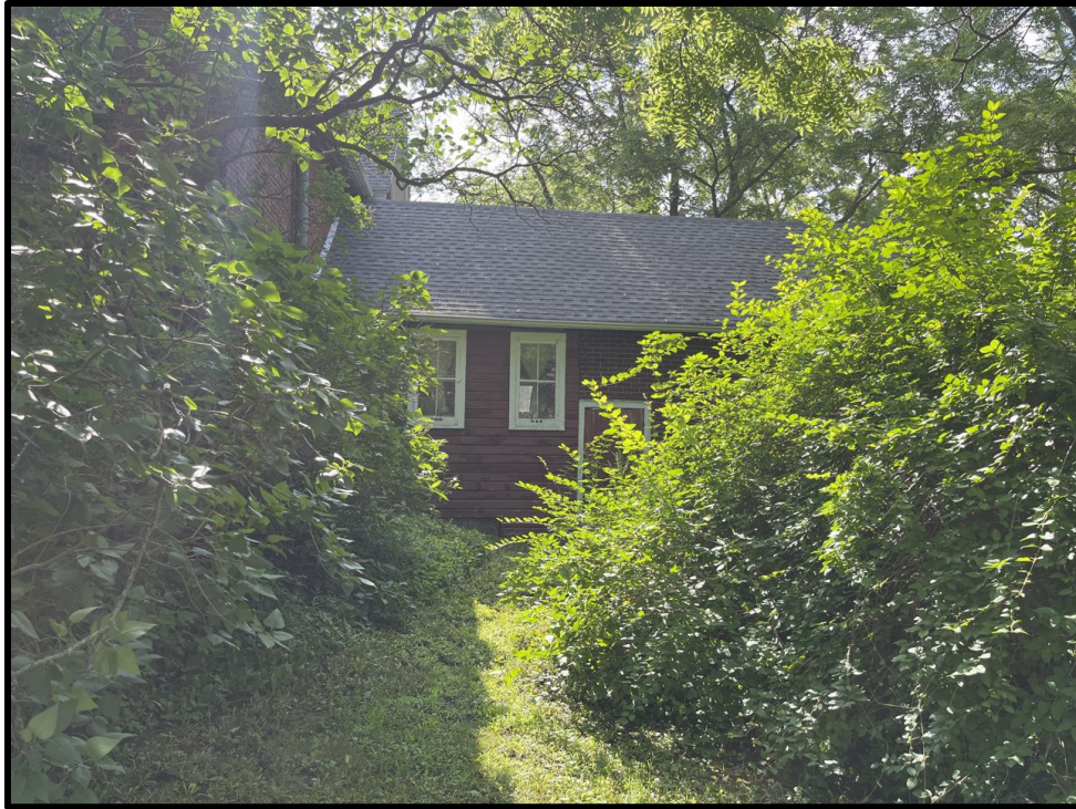
Image 17: Addition - Northwest Elevation of 5187 Sherkston Road (Photo taken on July 21, 2023; Facing Northeast)
