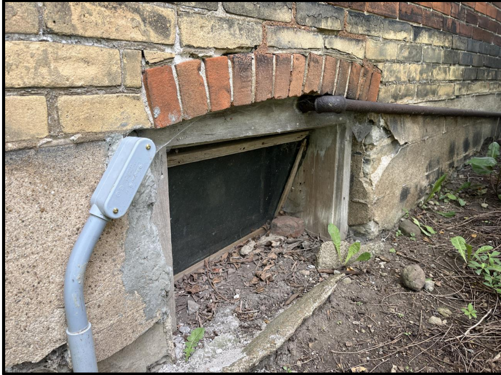
Image 11: Detail of Basement Window and Foundation of 5187 Sherkeston Road (Photo taken on July 21, 2023; Facing Northwest)
