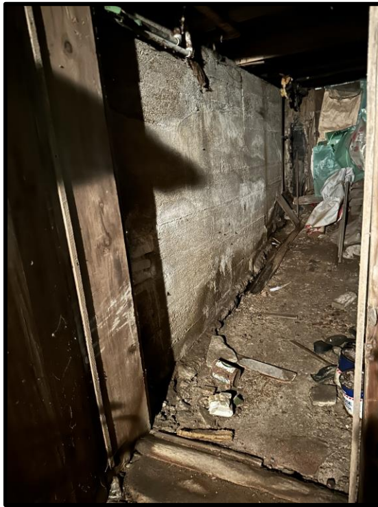
Image 54: Interior – Basement - Detail of Poured in Place Concrete Walls – 5187 Sherkston Road (Photo taken on July 21, 2023)
