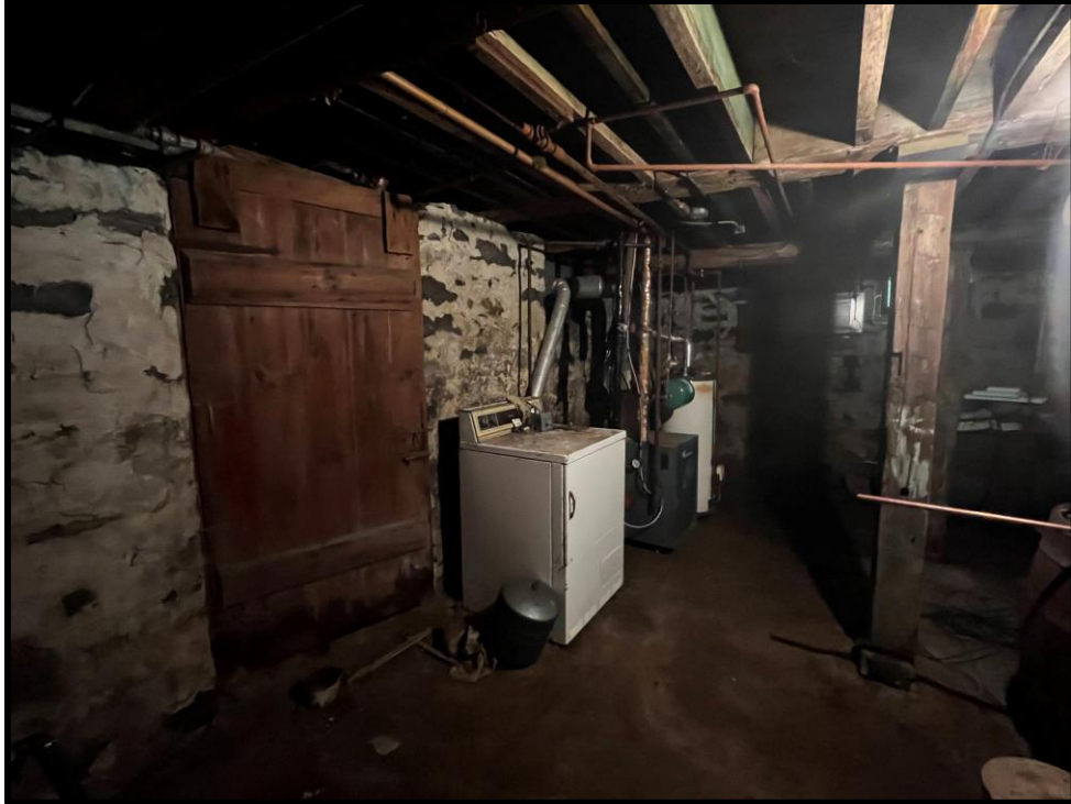
Image 53: Interior – Basement - Detail of Poured Stone Foundation Walls – 5187 Sherkston Road (Photo taken on July 21, 2023)
