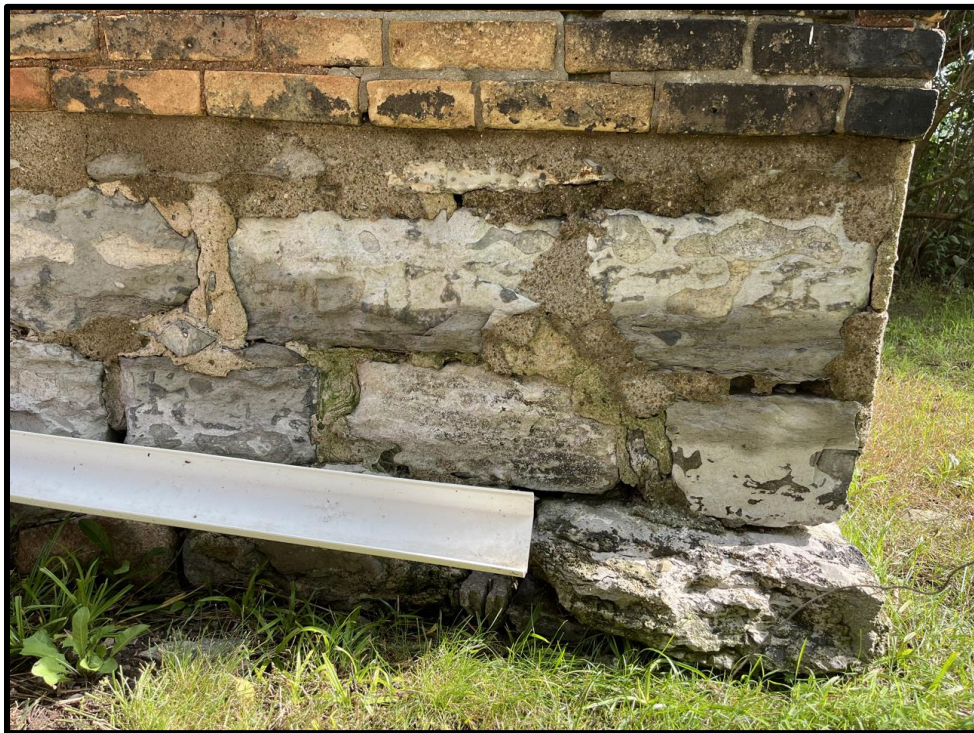
Image 12: Detail of Foundation at South Corner of 5187 Sherkeston Road (Photo taken on July 21, 2023; Facing West)
