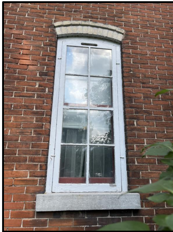
Image 10: Detail of Window with Buff Brick Voussoirs and Dressed Stone Sill of 5187 Sherkston Road (Photo taken on July 21, 2023; Facing Northwest)
