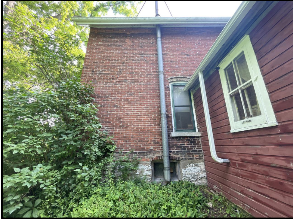
Image 15: Main House - Southwest Elevation of 5187 Sherkston Road (Photo taken on July 21, 2023; Facing Northeast)
